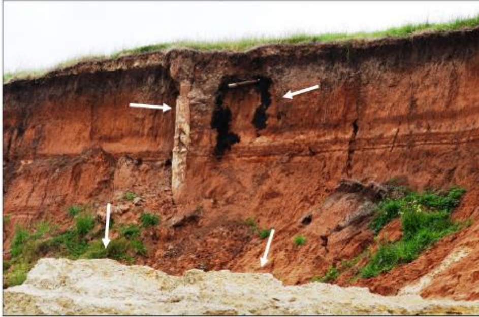
Figure (above). Well casing and other oil and gas activities that have become exposed by erosion along the Brazos River. Note the dark staining around abandoned infrastructure and well casing near the ground surface, and former waste pit (pale white sediment) eroded into the river at the bottom of the photograph, creating potential hazards to human and environmental health. Courtesy of Lower Brazos Riverwatch.
